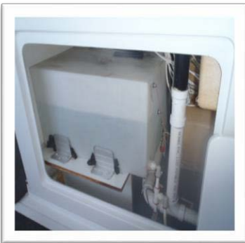
Potable Water Tank
