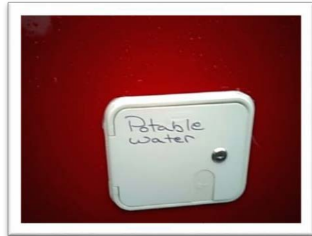
Potable Water Inlet
