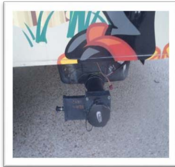
Liquid Waste Connection
